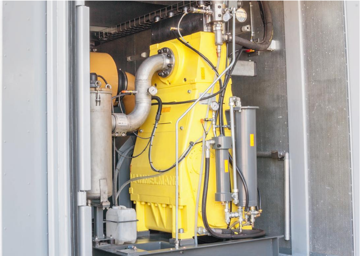
Stationary diesel unit in a soundproof container
